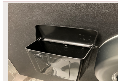
Figure 2. Sanitary disposal bin without a liner
